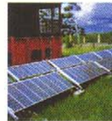
Solar Photovoltaic / Wind Power Systems
